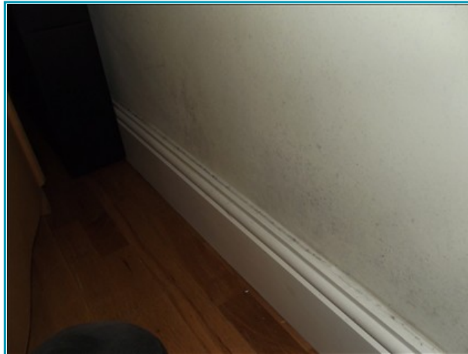
Mould spores to exterior wall in under stairs area.
