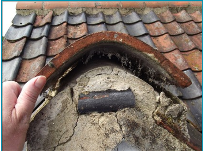
Loose ridge tile above rear Entrance Door.
