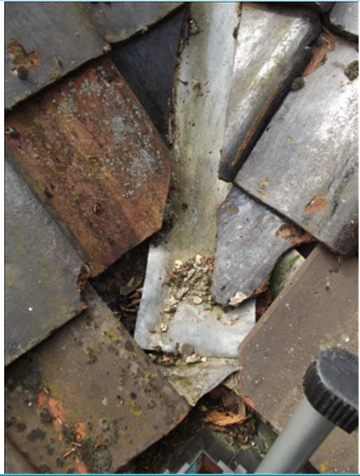
Roof valley not finished at bottom with tiles missing above rear Entrance Door.
