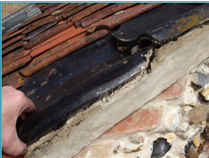
Loose verge tile to the rear single storey gable end.
