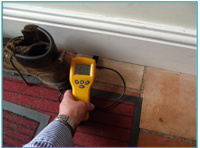
Damp to skirtings in rear Lobby.
