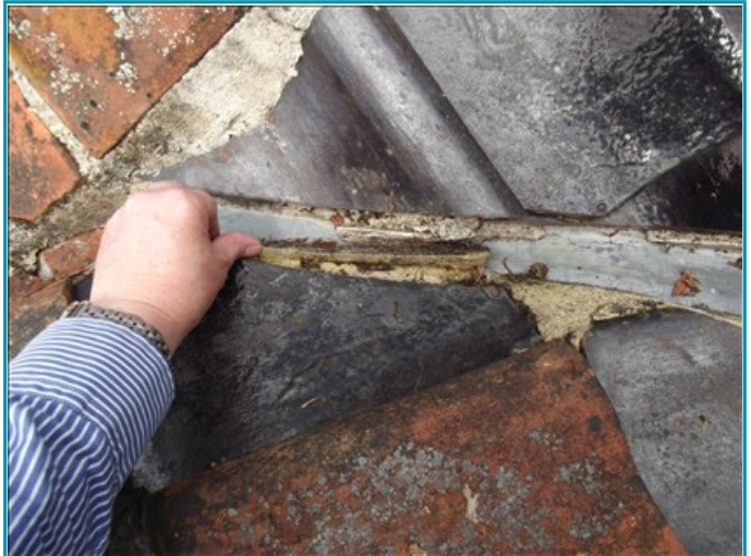
Loose cement parging to roof valley.
