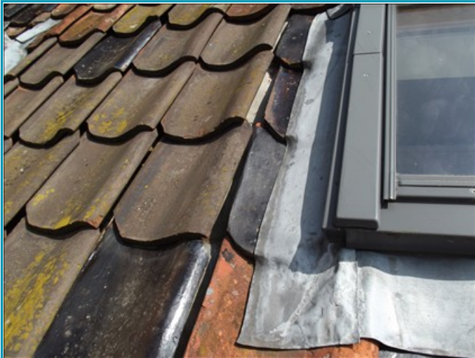
Roof tiles set out so badly they are not over lapping.
