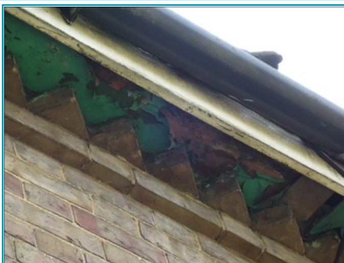
Rot to softwood soffit on front elevation.
