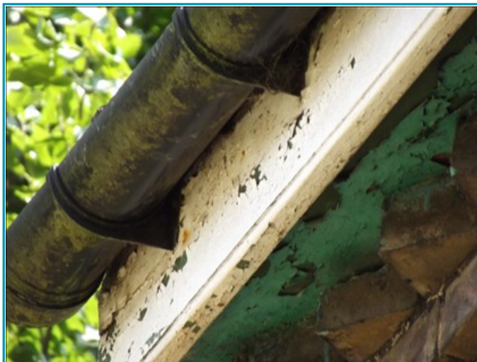
Flaking paintwork to front elevation softwood fascias and soffit.
