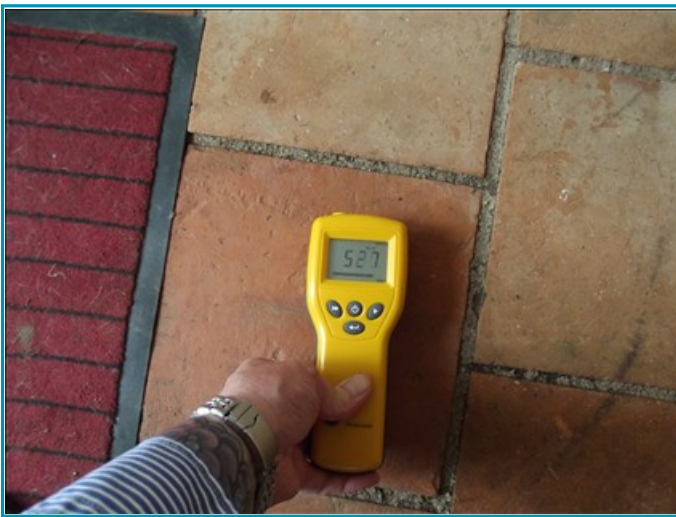
Damp to clay pavement floor tiles in rear Lobby.
