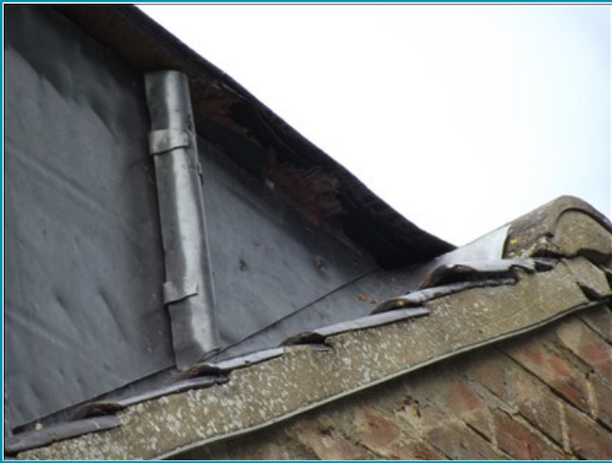
No fascia or aris cut to the left hand side of the rear dormer.
