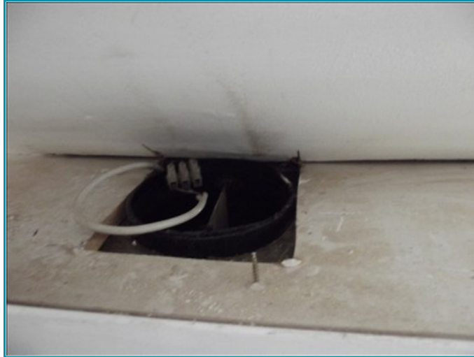
Cooker hood extractor fan is not connected to the exterior.
