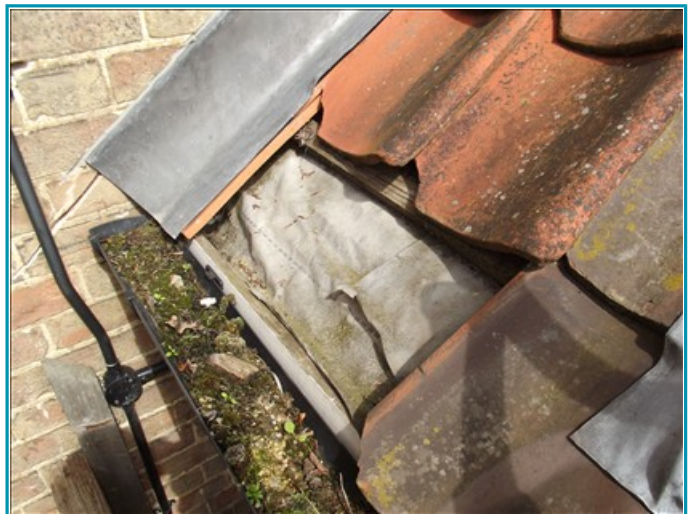
Two roof tile missing from the rear roof elevation over the Breakfast room.
