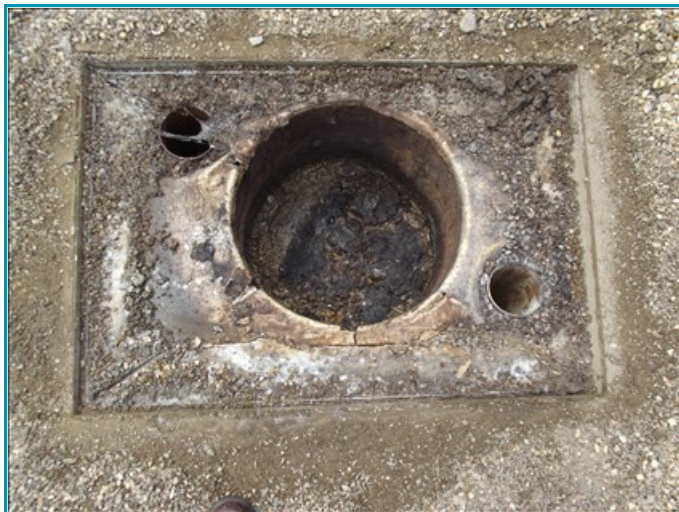
Septic tank full.
